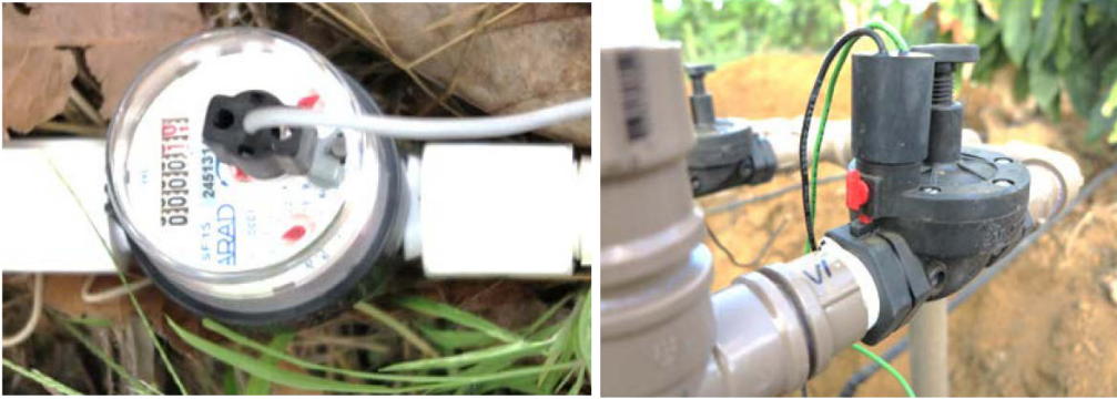
Figure 68: Flow meter and electric valves for automated irrigation.
