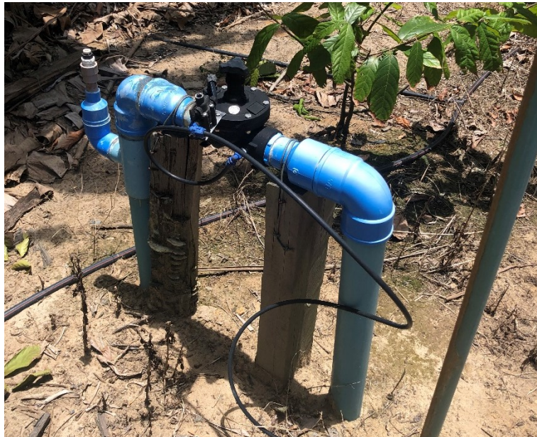
flowmeter & electric valve
