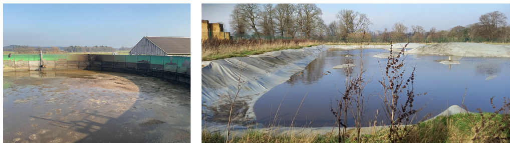
Figure 7. Slurry tank (left) and lagoon containing approximately 8 million litres of manure (right), UK dairy farm. Manure lagoon is covered by white geomembrane liner cover, with vents. Rainwater has accumulated over the canopy. Large upward bulges (whales) may be lifted up by underlying volumes of methane.
