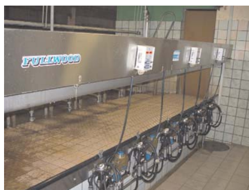
Salle de traite side by side
